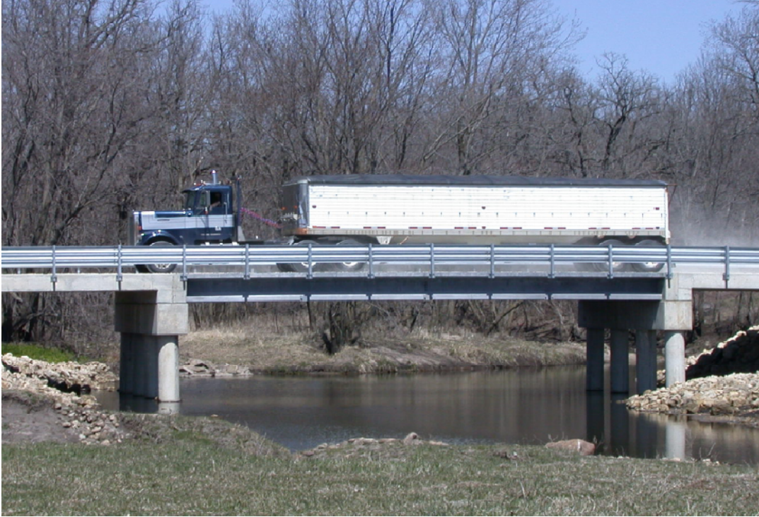
Figure 2.12: View of the Completed UHPC Jakway Bridge in Buchanan County, Iowa (Bierwagen, 2009)
