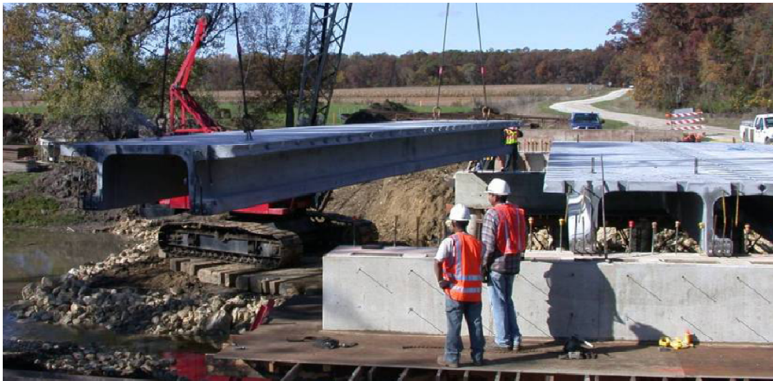
Figure 2.11: Installation of the Second Generation UHPC Pi-Girder on the Jakway Bridge in Buchanan County, Iowa (Bierwagen, 2009)
